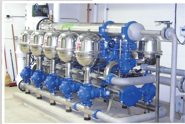
Lake Water Filtration System
