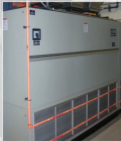
Computer Room Unit
