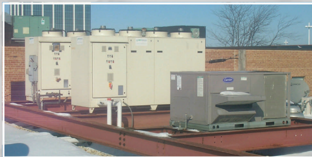
Rooftop Heating and Cooling Equipment
